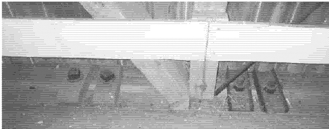
Figure 8. Detail of U-bolt connection of girders to the bottom chord (older connection on left)
